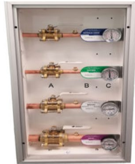
Medical Gas Valves
